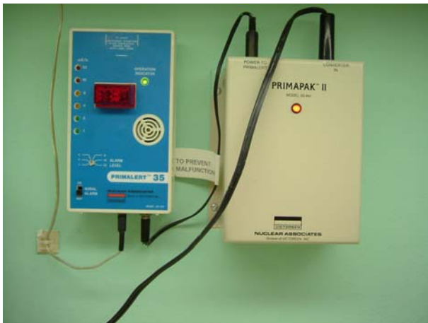
Figure 6 Exposure rate meter mounted on a wall in the treatment room so as to be visible from the entrance way.
